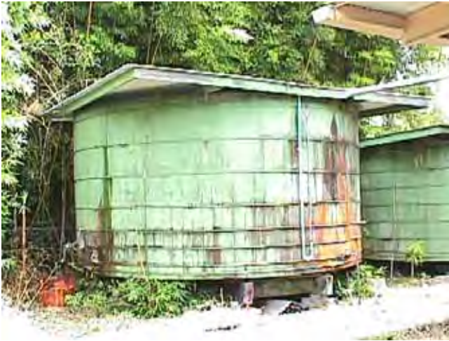
An older redwood tank. Beware of redwood tanks that were painted on the inside with lead paint to discourage algae.
