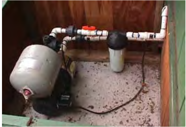
A small but typical electric pump. The pump sits below a pressure chamber. A coarse filter hanging from the inlet pipe filters the water before it enters the house.
