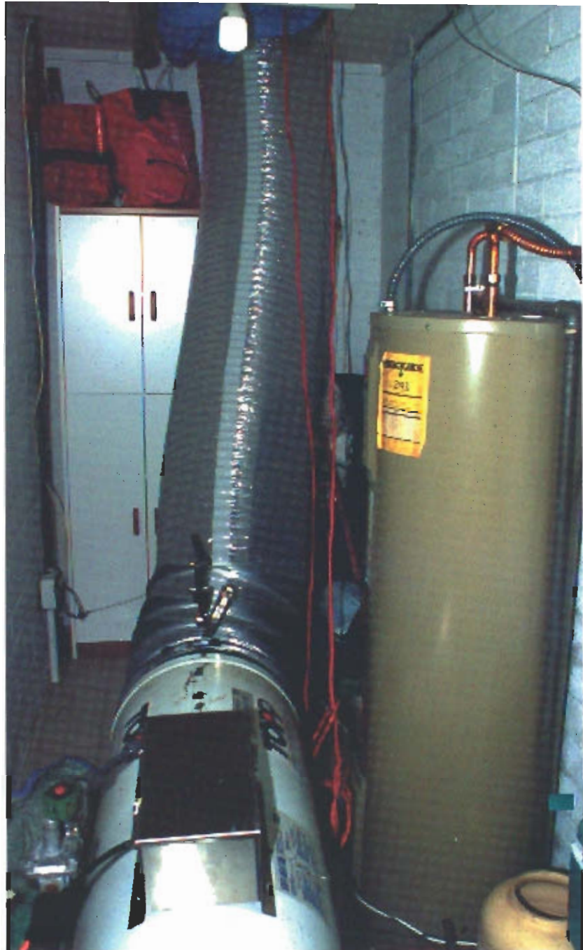
The TPE process uses large gas space heaters that blow heated air into a structure to raise and maintain the ambient temperature of the structure.
