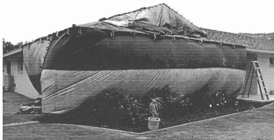
Fig. 4. Side view of the high temperature treatment done at Hawaii Kai, Oahu, 10 May 1995.
