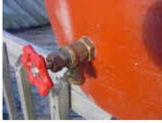
Fig. 3: Drain spigot at bottom of rain barrel
