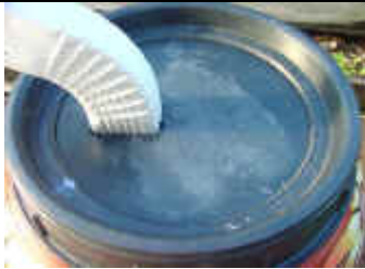
Fig. 4: Gutter downspout into top of rain barrel (unscreened)
