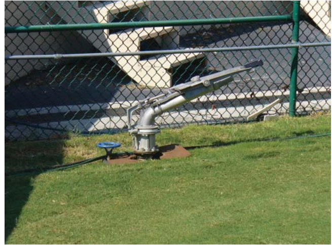
3. Aboveground irrigation gun used for athletic field irrigation
